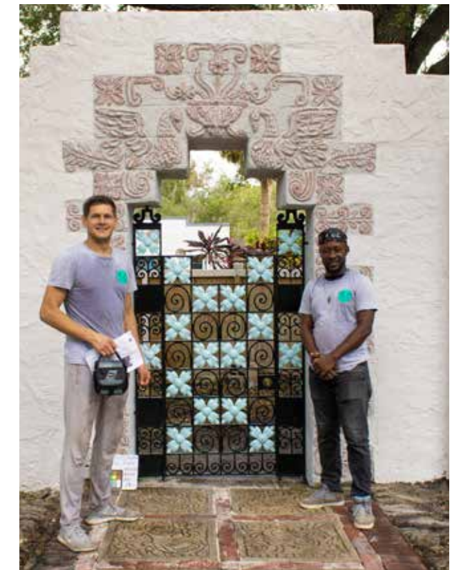
Our Main Garden gate restoration is complete! Pictured are team members from RLA Conservation (out of Miami), who oversaw the process of historic restoration.
